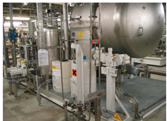
Figure 1.1: Potable water system with evaporator, scale inhibitor tank, chlorine tank, alkalizing filter and UV units (Photo: Eyvind Andersen)
