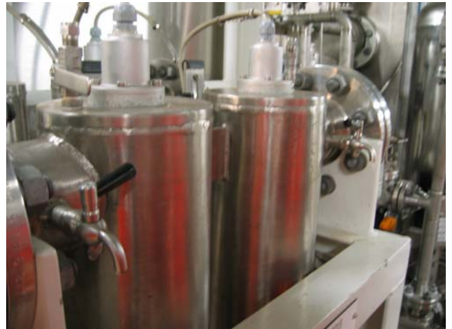
Figure 8.5: UV unit with test taps before and after disinfection (Photo: Eyvind Andersen)
