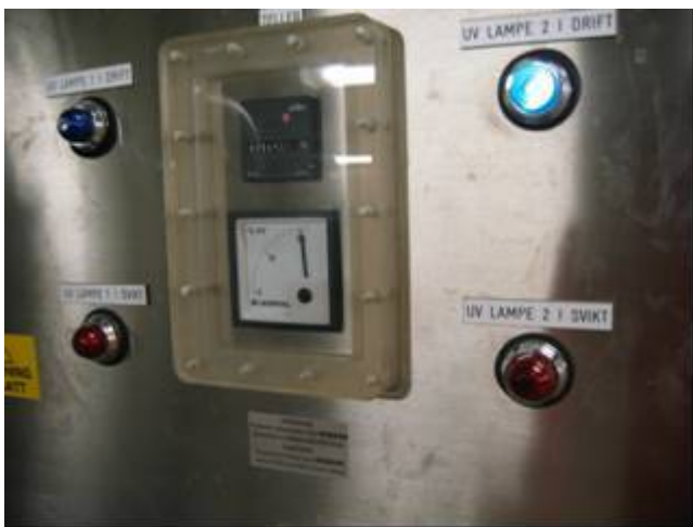
Figure 8.6: An UV unit control panel with two UV radiation tubes. The blue light indicates that radiation tube number 2 is in operation and functioning. In the centre of the picture you can see a time recorder (black) and an UV intensity meter (Photo: Eyvind Andersen)
