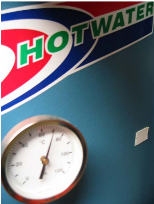
Figure 4.4: Problems with Legionella bacteria growth is avoided by keeping the hot water temperature high (Photo: Eyvind Andersen)
