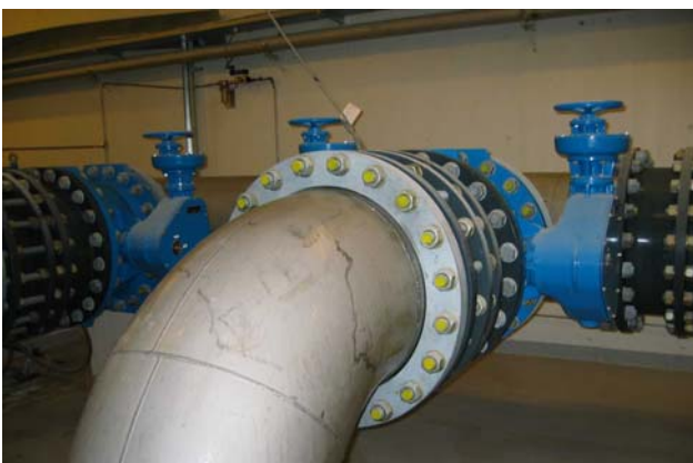
Figure 9.6: Pipes and valves in potable water systems vary in size and material. It is important that corrosion resistant materials and materials that do not encourage bacterial growth are chosen (Photo: Eyvind Andersen)
