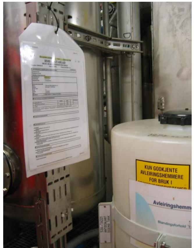
Figure 5.3: Sufficiently marked and secured tank for scale inhibitor (Photo: Eyvind Andersen)
