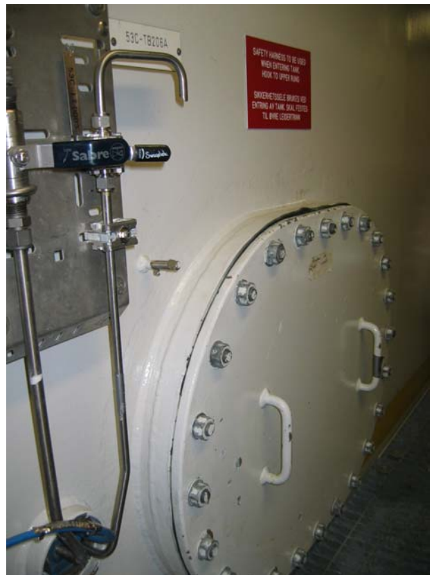
Figure 9.3: The picture shows a storage tank with easily reached test tap and an accessible manhole (Photo: Eyvind Andersen)
