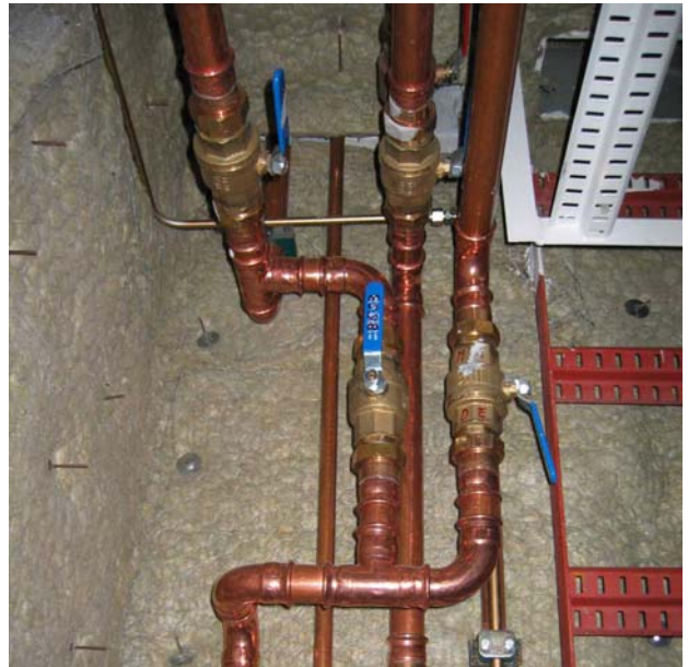
Figure 4.7: Corrosive water in copper pipes can result in too high copper content in the potable water (Photo: Bjørn Løfsgaard)
