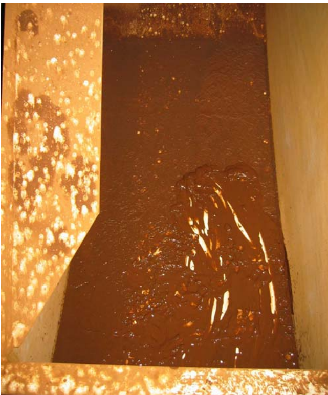
Figure 3.1: Demand for cleaning of tanks at least once a year is set to avoid situations illustrated in the picture above, where there is a layer of mud at the bottom of the tank. Such occurrences have to be handled as a non-conformity case. (Photo: Bjørn Løfsgaard)
