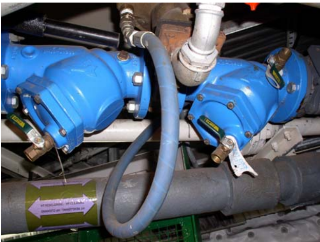
Figure 9.5: Other liquid carrying systems should not be supplied with potable water. If this can not be avoided, broken connections or double back-suction/back-flow protection, with drainage between the two systems, will give the best protection against contamination (Photo: Eyvind Andersen)
