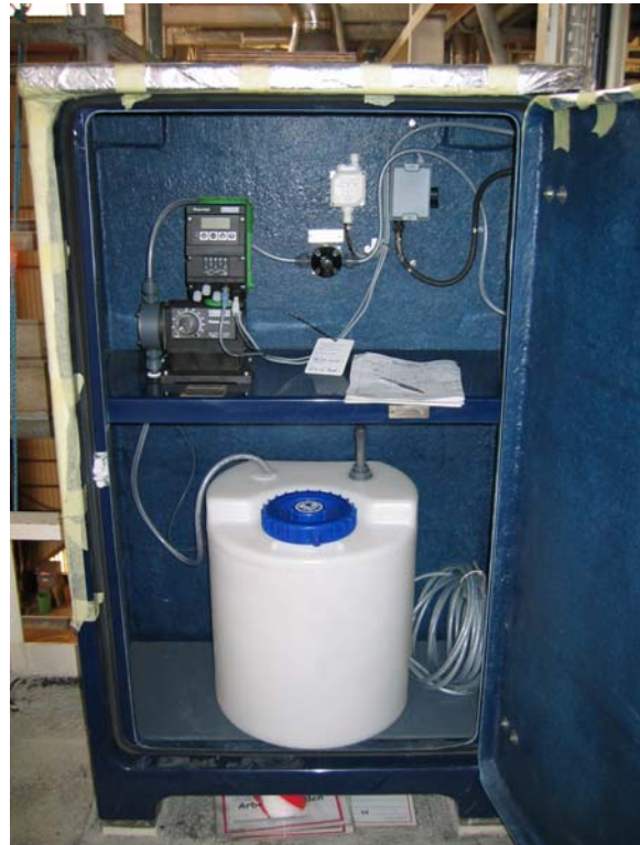
Figure 8.3: Flow meter controlled chlorination unit, safely placed in a cabinet (Photo: Bjørn Løfsgaard)
